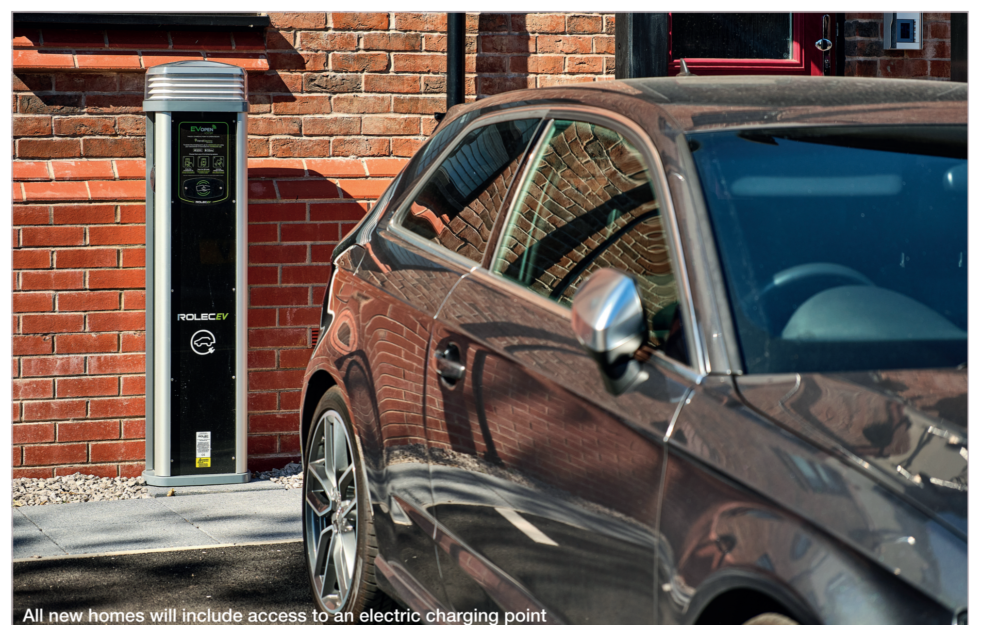
All new homes will include access to an electric charging point
